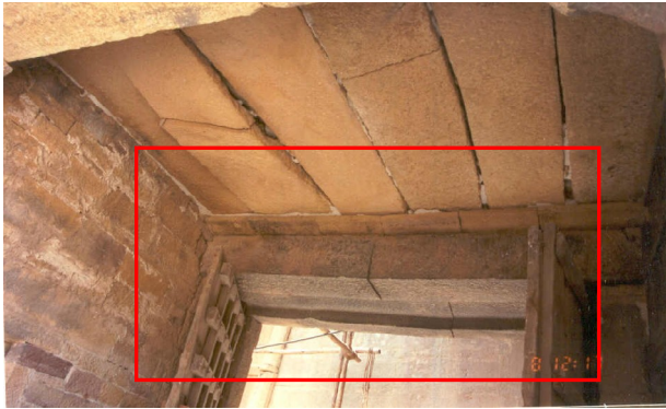
Sagging lintel and frame in the interior
