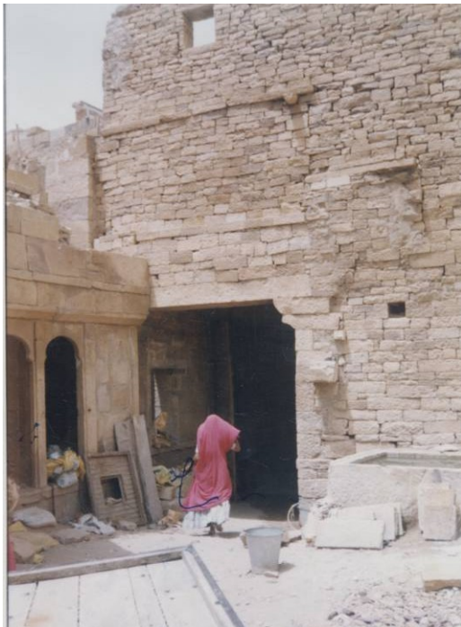
Wall over the gateway was in a dilapidated condition
