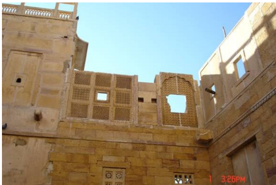
Decorative Jali work on the third floor over the Tambu Khana Chowk is being reconstructed, although the room has not been constructed as yet.
