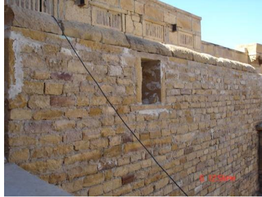
Edging of Parapet on First Floor has been done by chamfering the stone
