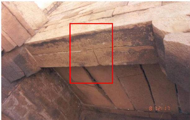
The stone slabs have been restored and neatly joined to form the gateway
