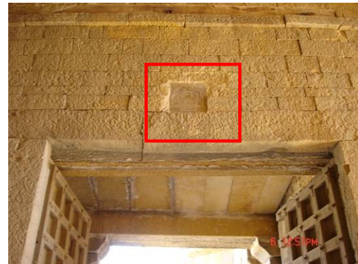
Wooden doorframe and stone lintel have been retained but reassembled, to remove faults
