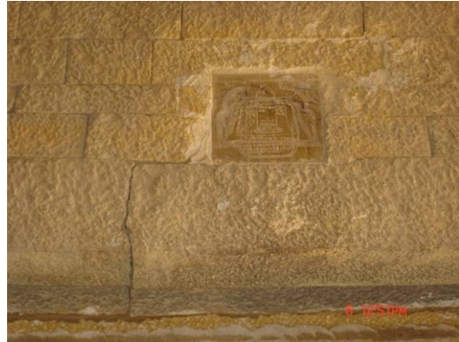
Detail of Historic carving over gateway which has been restored and retained in its original position
