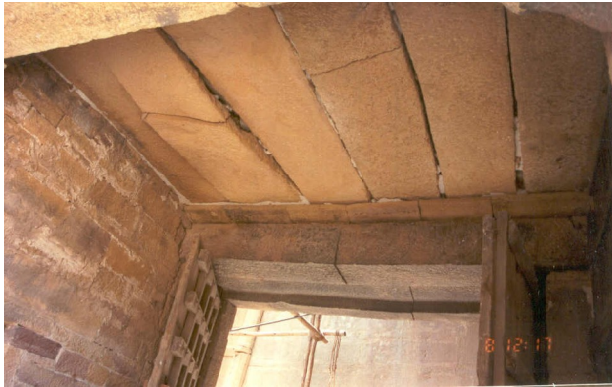
The stone slabs were broken and disjointed under the tremendous load
