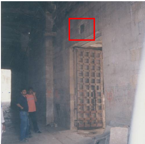
Sagging lintel and frame
