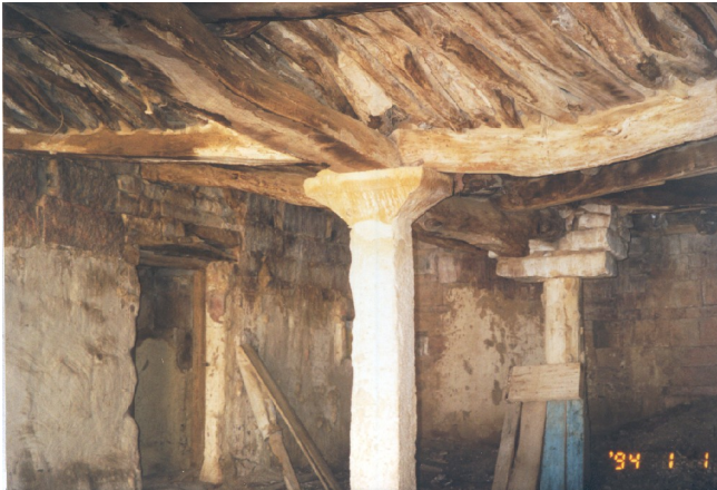
Wooden members were sagging under the load, and were badly damaged
